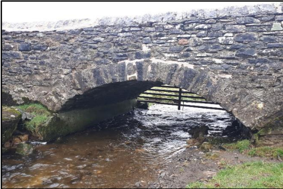
Damaged bridge prior to commencement.
