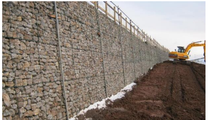
The finished wall with over 4000t of gabion stone. The scaffolding on the front was used to protect operatives from falls from height.
