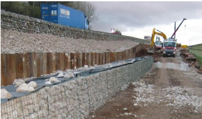
The first layer of baskets installed on a sub base foundation, and behind them some of the sacrificed steel piles.
