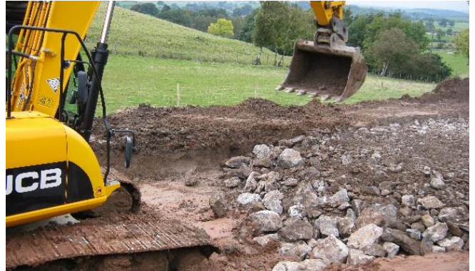
The first job was to install a haul road to allow access to the site. The road went over wet ground and was benched into the embankment.
