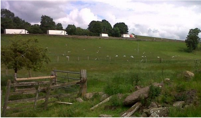
The original sandstone retaining wall was subsiding and the road was likely to give way.
